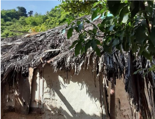
Inadequate Thatched Roof in Platon
