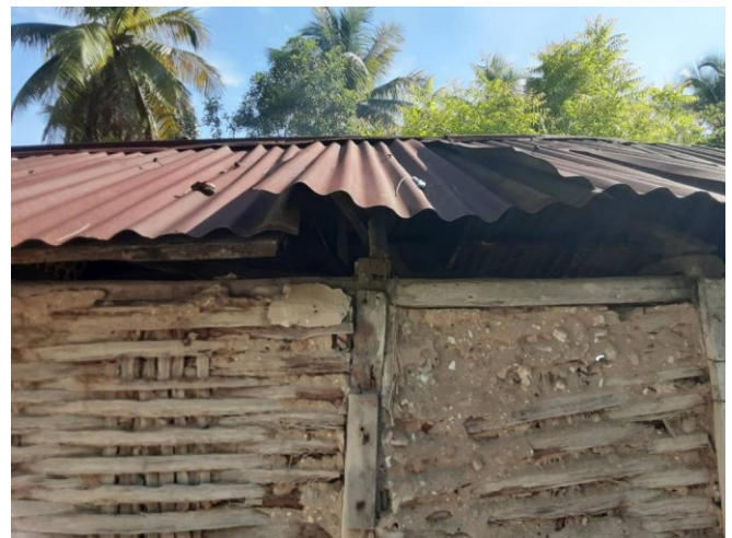
Platon House with leaking roof
