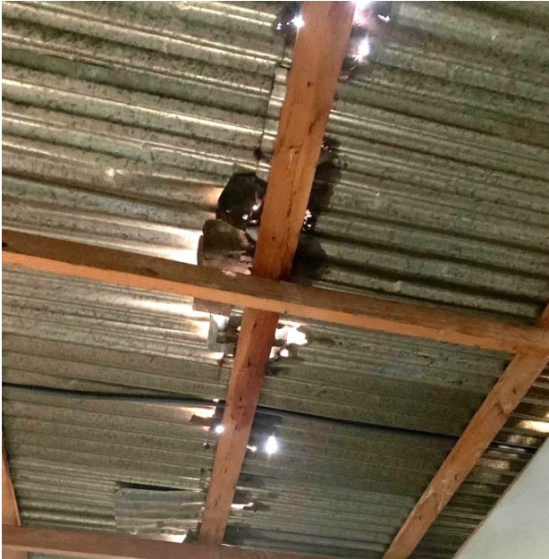
Christella Julsaint's Leaking Roof
