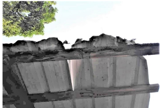
Porch Roof Damage
