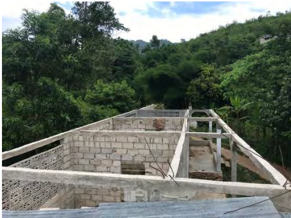
The above structure will be rebuilt, floored, roofed and modified. The advice of the NCSU Architecture Department is being sought.
